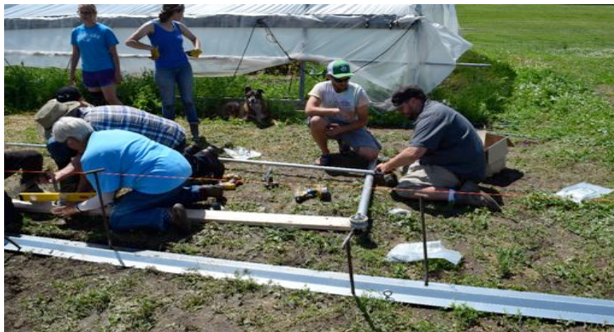
The work crew gets down to the nitty gritty of construction of a moveable high tunnel at Johnson County Community College. Photo from Tom Buller.
