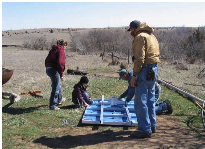
Michael shows his family and friends how to assemble the solar panel for the pump. His family and friends were instrumental in the process of adding the solar-powered pump, waterlines and three tanks to Michael's pasture. Submitted Photo
