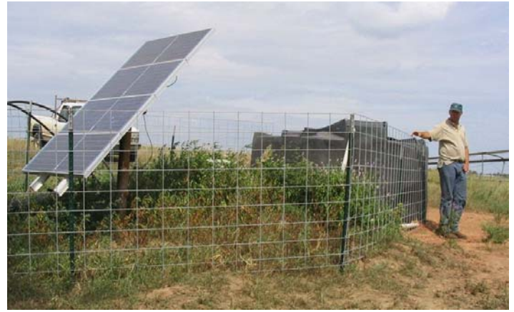
Michael Scheer uses a solar powered pump to bring water into a 4,000 gallon supply tank. Michael implemented the pump and tank using CWFP cost-share funds. Photo by Mary Howell
