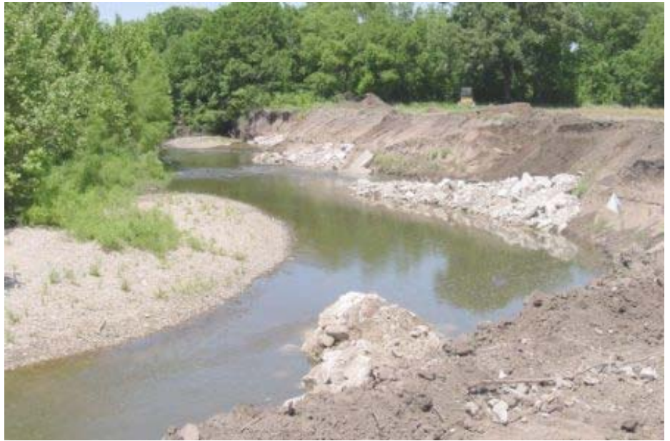
Don was concerned about the amount of erosion along the Little Walnut River. The State Conservation Commission, the Kansas Alliance for Wetlands and Streams (KAWS) and the Watershed Institute all worked together to plan and install rock vanes along the river to reduce erosion. Submitted Photo
